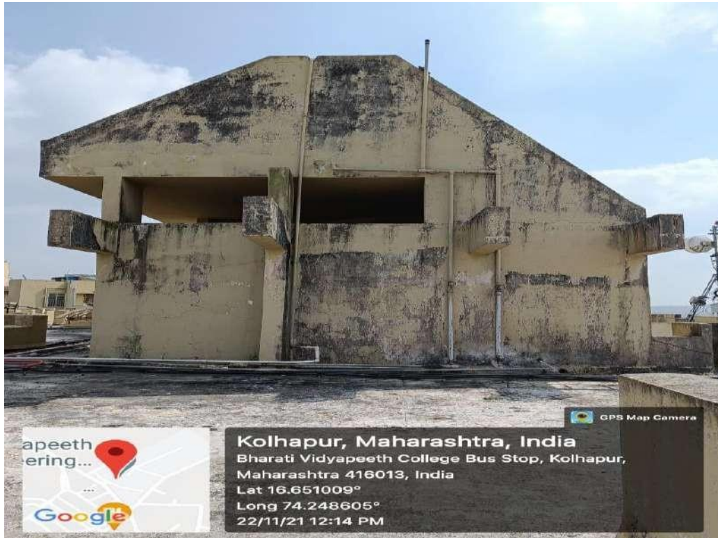
Main building cement water tank
