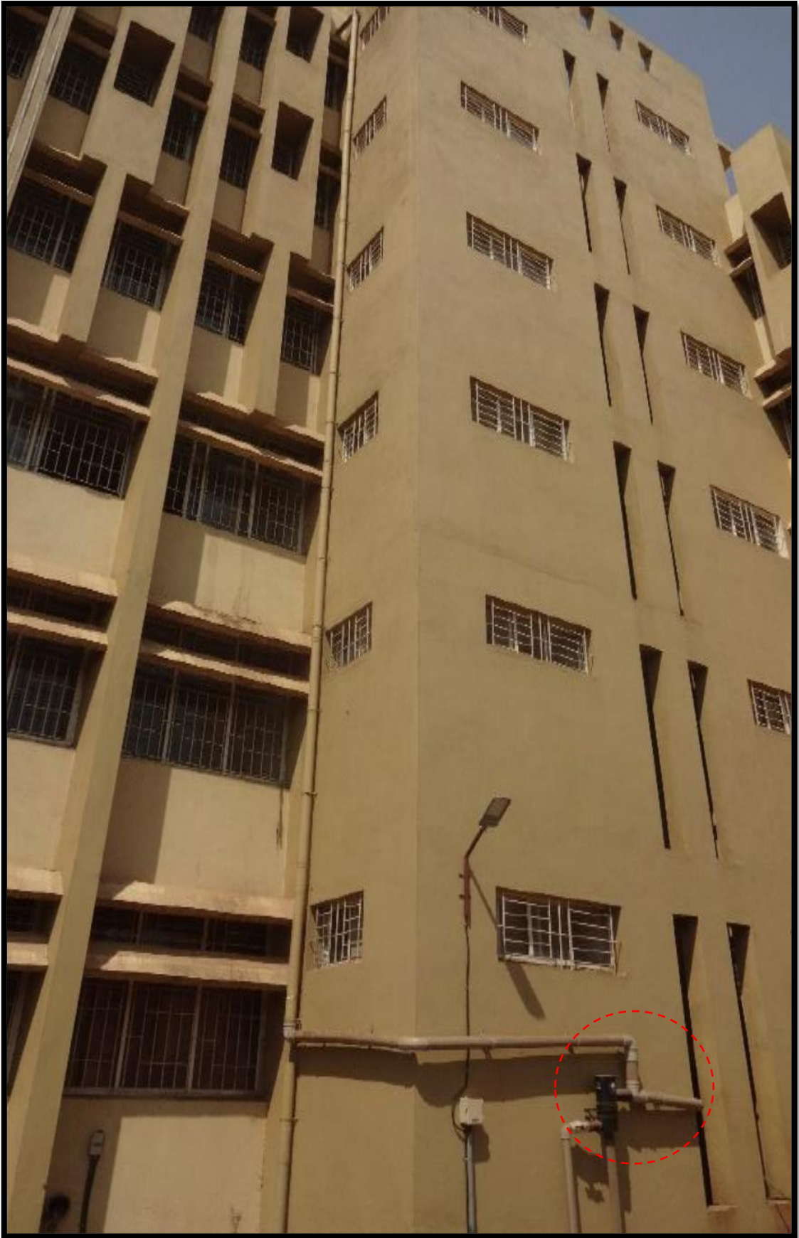
Rain Water Harvesting system
