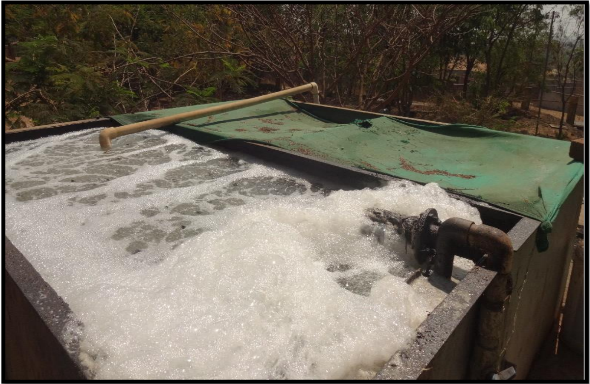
Decentralized Waste Water Treatment Plant during operation
