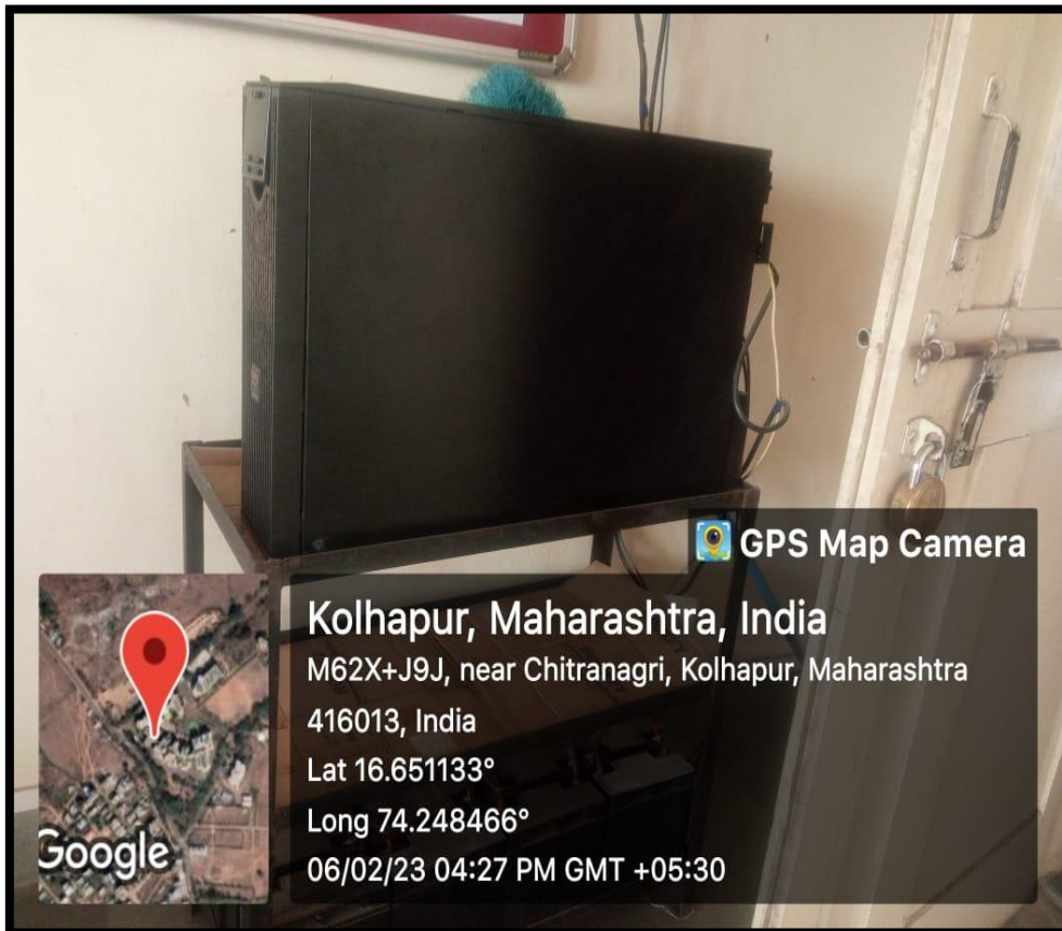
Uninterruptible Power Supply (UPS)
